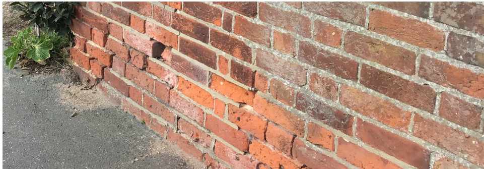
Figure 44 Damaged brick boundary wall to the row of cottages
