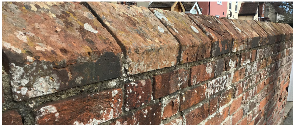
Figure 28 Brick wall with triangular section copings to the cottages along Thorpe Road
